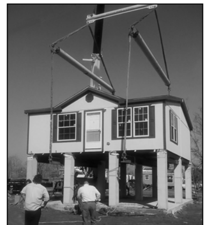
Above: Disaster recovery funds in Sabine Pass help to elevate a home to make it better able to weather future storms.
